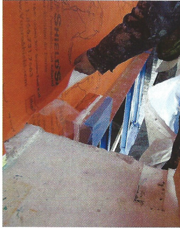
An installer from Prospect Waterproofing Co. removes the release paper from the self-adhered membrane, lapping over a penetration in shingle fashion, to maintain continuity of the air barrier system. Photo courtesy of Jim Glaze, Thamco Inc.
