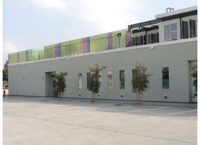
3,500 sq. ft. of WrapShield HS Water Resistive Vapor Permeable Air Barrier Membrane was installed under stucco.
